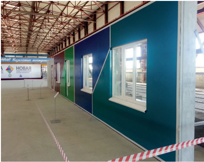
Ready for assembly on the building site: precast concrete side walls with already installed windows.
