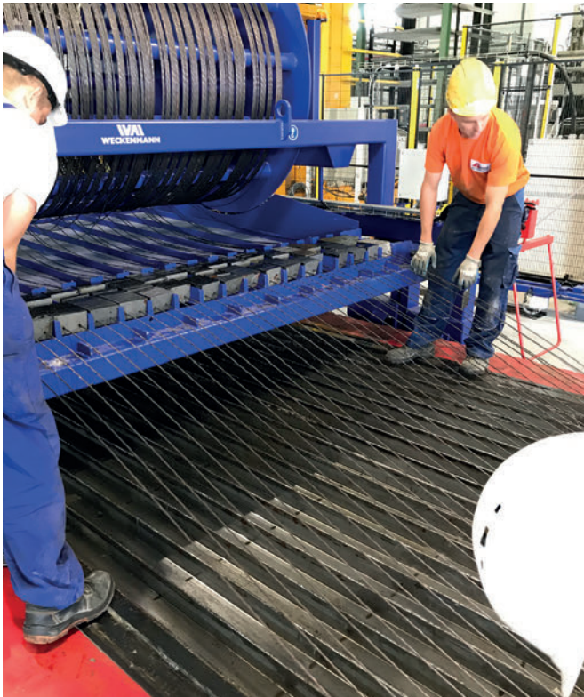
The transport drum for prestressing wires
